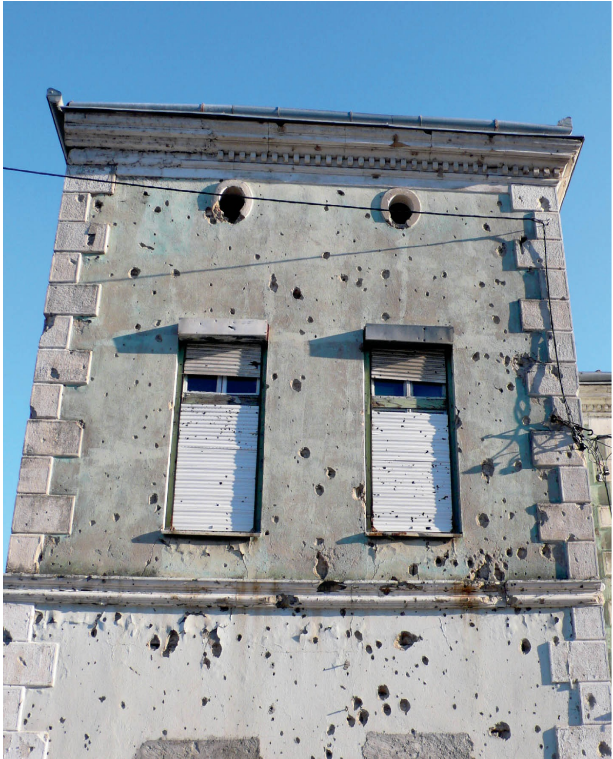
Destructive Points Never underestimate the power of a point. This damaged facade was photographed in the war-torn city of Mostar, on the Balkan Peninsula in Bosnia and Herzegovina. Nancy Froehlich.
