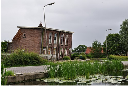
Inadequate foundations in muddy soils below sea level caused these houses in the Netherlands to subside .
